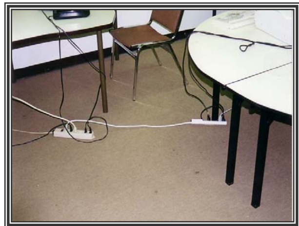
Strings of extension cords and extension cords connected to extension cords or power strips are not allowed under fire codes.
